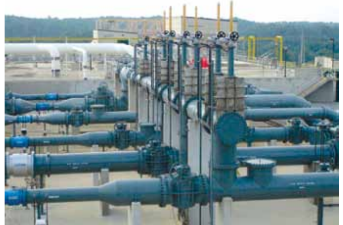
30", 36" & 42" Solid SS Bonneted Knife Gates, 50 psi, Wastewater Treatment Plant Gwinnett County, GA
