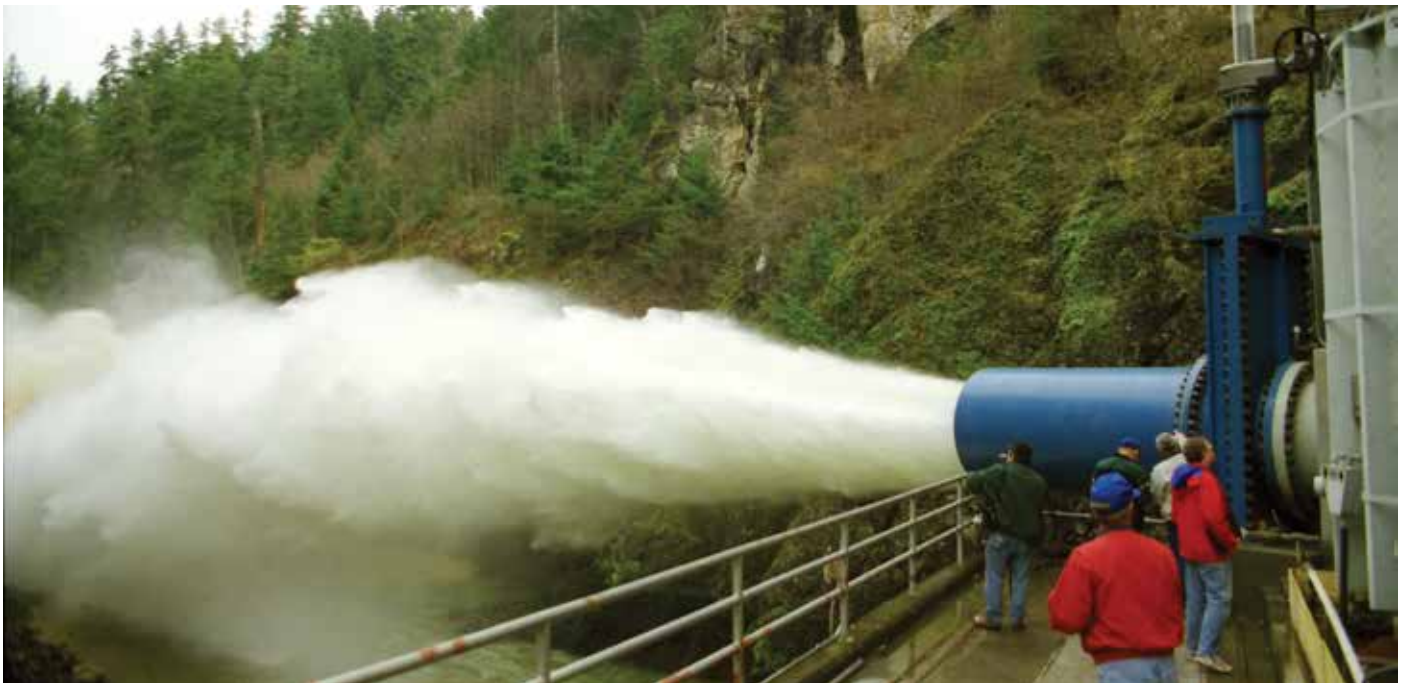
This 42" Hilton Jet Flow Gate Valve is installed at LaGrande Dam near Tacoma, Washington.
