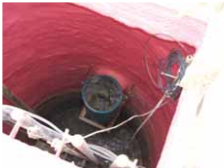
Vortex Flow operating in a pumping station wet well, Jacksonville, Florida.
