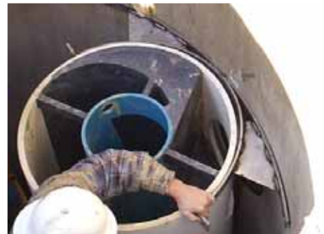
Securing Vortex Flow unit, Burlington, Kentucky.
