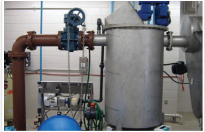
Chemical Mixing System.
