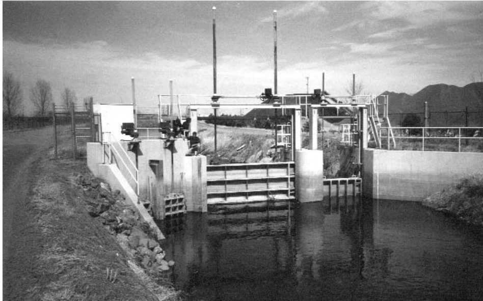
Tandem electrically actuated roller gates.
